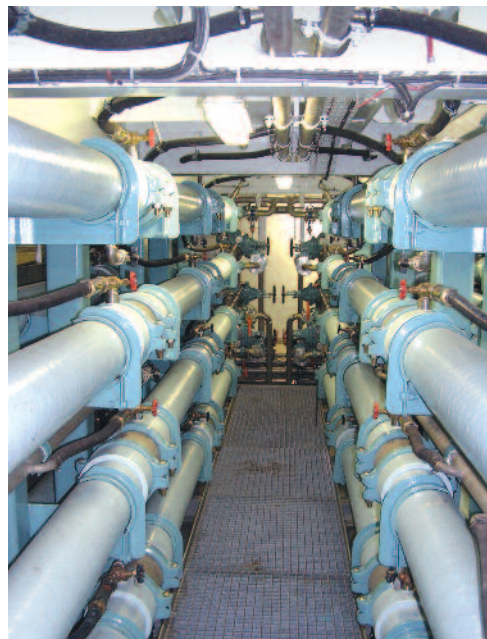
Typical MBR installation
