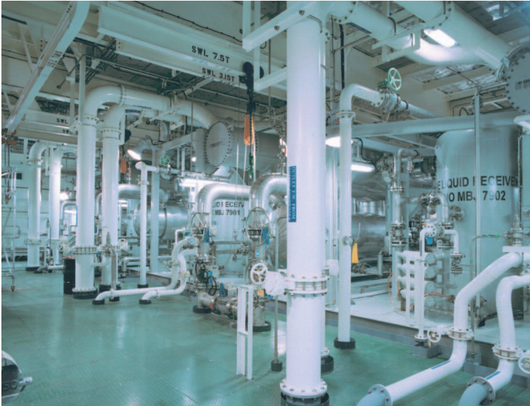
Cooling plant installation onboard 'Sanha' LPG-FPSO
