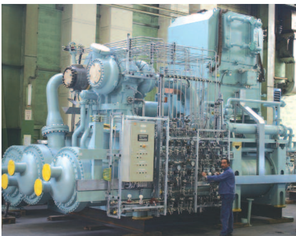
Typical N2-compressor with coolers (one expander)
