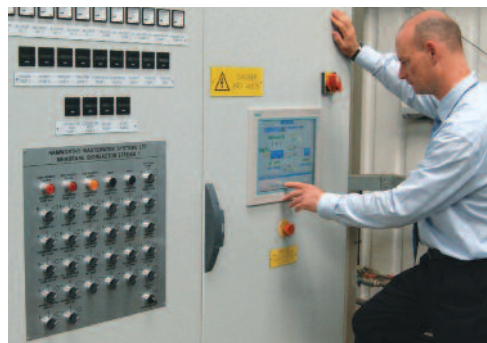
MBR control panel
