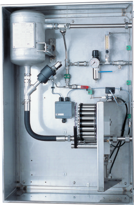
FLARE GAS IGNITION CABINET FOR AUTOMATIC OPERATION
