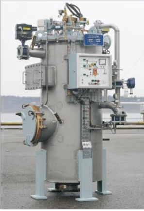
Moss Topping Up Generator
