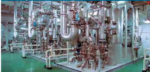
LPG reliquefaction system on board the Sahna LPG FPSO
