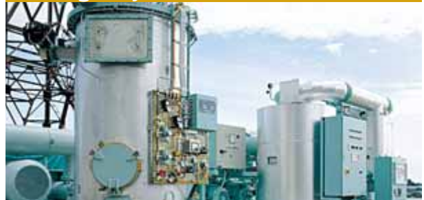
Inert gas systems on the quay side at Hamworthy's Moss facility
