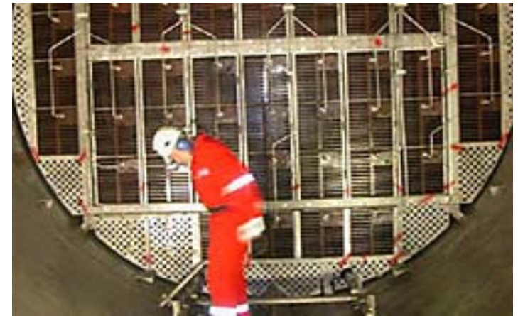
Hamworthy T&P's VIEC oil separation system
